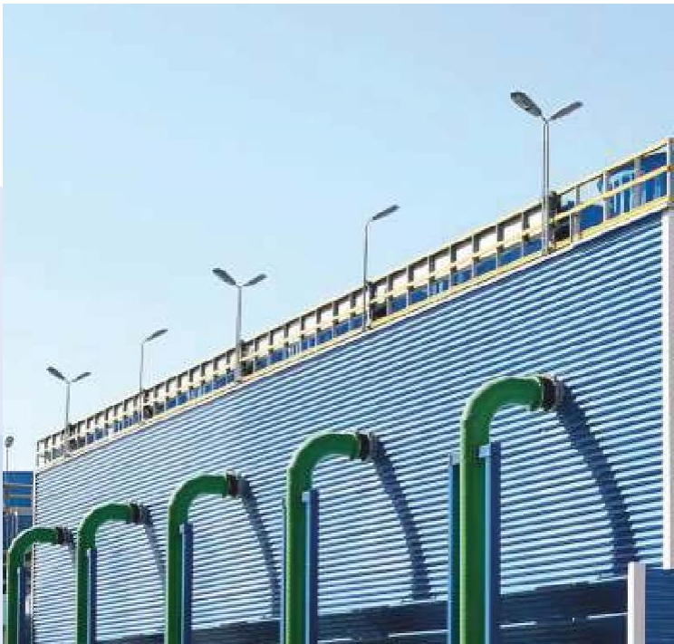
COOLING TOWER AREA
